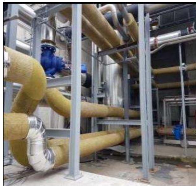
Turbine Integral Insulation
